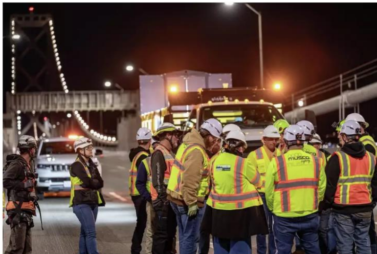
Crews started installing 50,000 custom-engineered LED lights on the Western span of the Bay Bridge this week, marking the first step in bringing the beloved Bay Lights art installation back to the Bay Area skyline after nearly two years of darkness. Ken Chan/Illuminate
